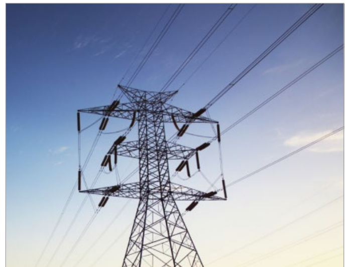
Photo: U.S. Department of Energy
